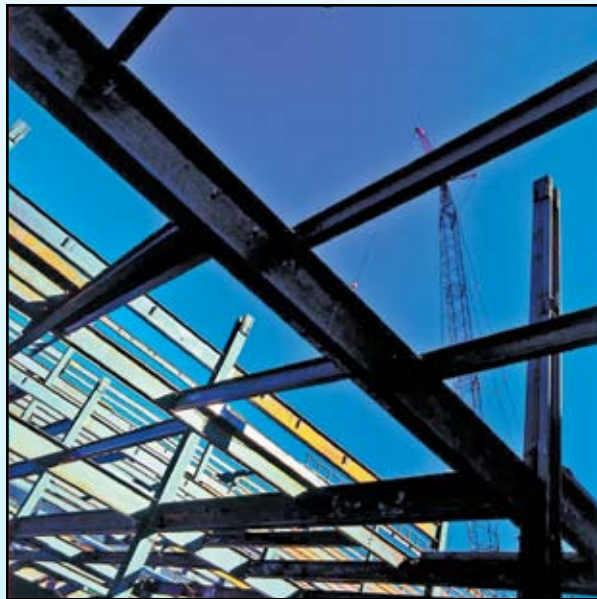
Using Constructability principles, the Mercy Heart Center Design/Build team shaved 16 weeks from the schedule and 140 tons of steel from the structure of the four-story, 144,000 square foot facility.
