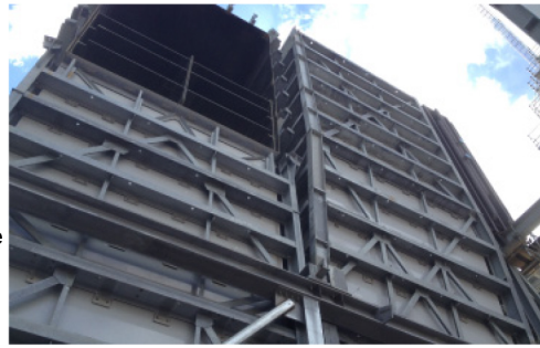
The steel skeleton was designed to provide strength and stiffness for the duct, while allowing for thermal expansion of the reinforced fiberglass.
