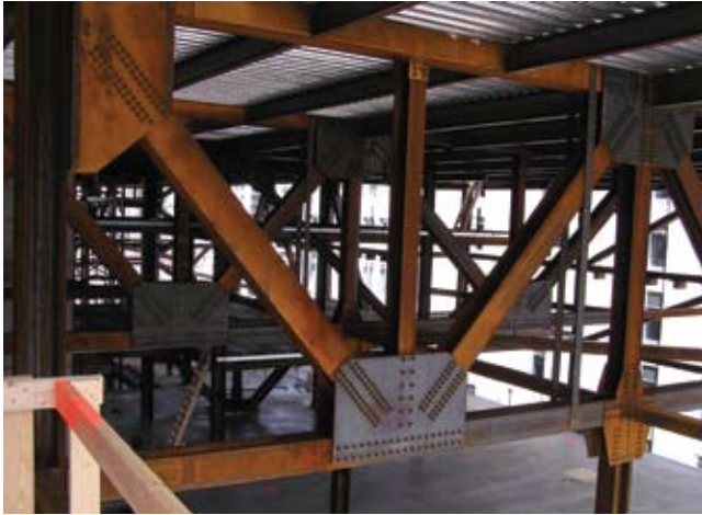
Ten transfer trusses housed in the hospital's 10th mechanical space reduce the number of columns on the first level freeing up space.
