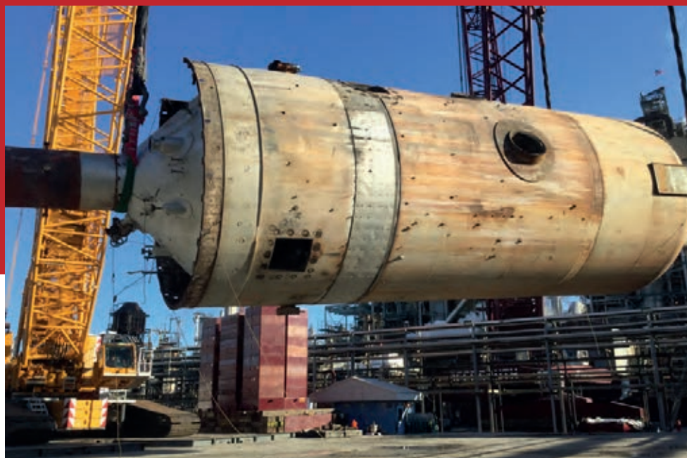
The 1940s-era reactor weighed 850,000 pounds and required lifting lugs and tailing rigging for the lift and laydown of the old reactor and installation of the new reactor.
