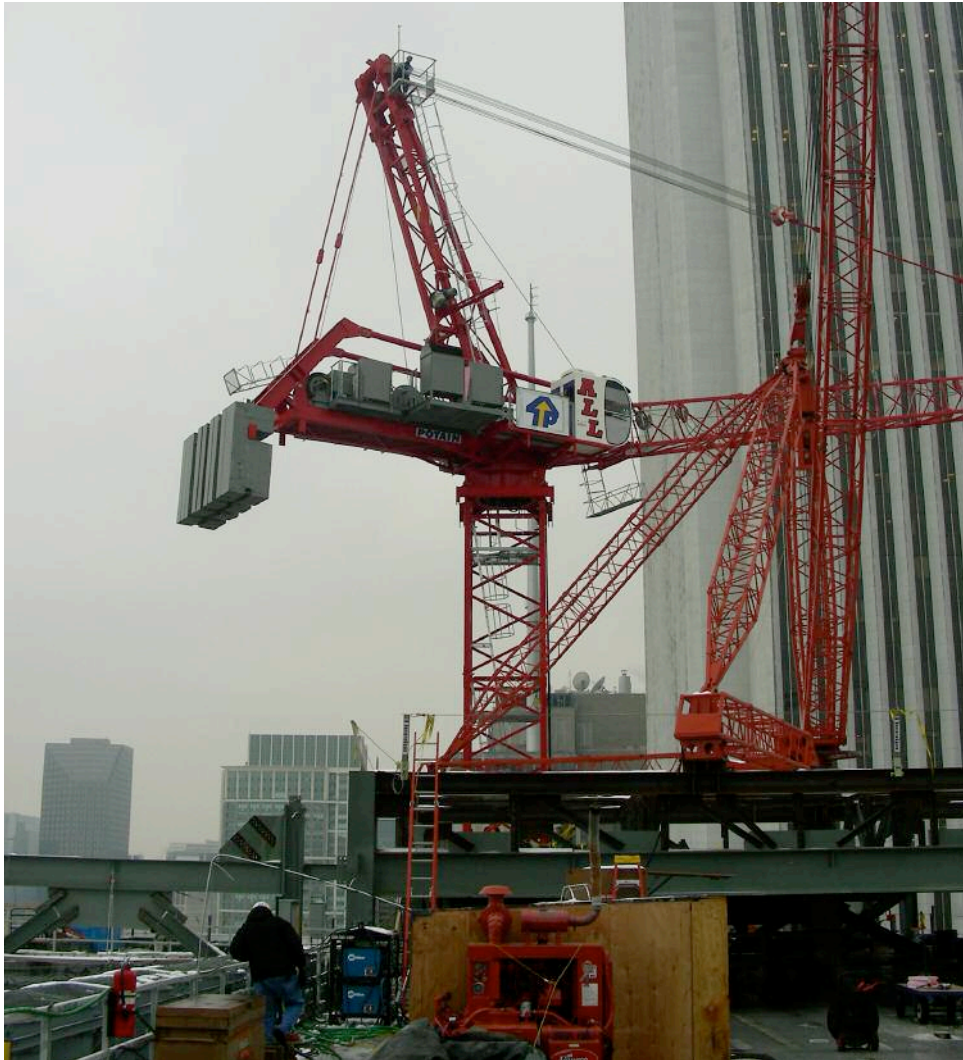
The Potain MD605E works alongside the larger of the two derricks, the Timberland SD 35-100. Both crane and derrick were mounted on a lattice of temporary structural steel supports.
