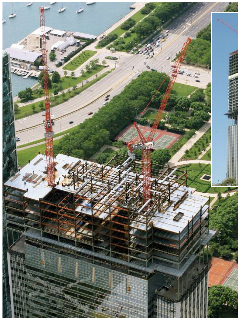
Above and left: Two Potain MR 605Bs, installed by derricks, work 400ft high (122m) to extend a Chicago skyscraper. Without using girders, the job of erecting the tower cranes would have taken 600ft (182m) of crane boom.
