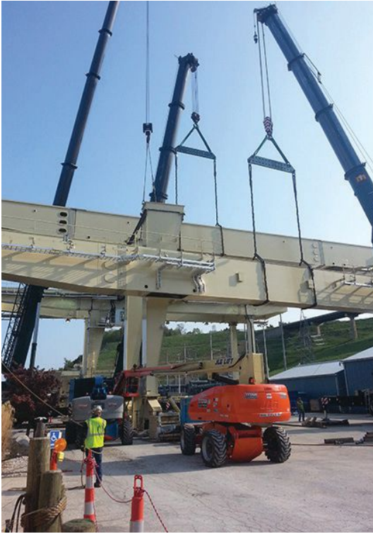
above: Lift beams were used for gantry crane erection at the Consumers Energy Pumped Storage Hydroelectric Plant project in Ludington, Mich.
